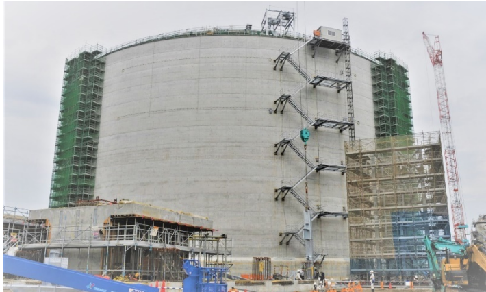
Building an LNG tank, the largest of its kind in Japan, on the premises of Ehime Works
