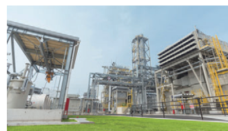
Niihama North Gas-Fired Power Plant
