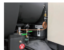
HFO (R1233zd) refrigeration equipment
