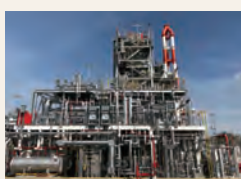
Pilot facility to produce ethylene from renewable ethanol
