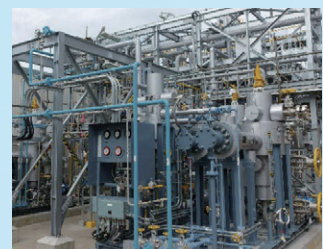
Pilot facilities manufacturing methanol from CO 2
