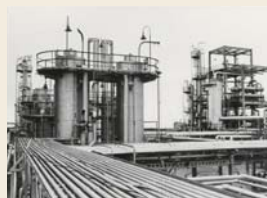
Ethylene Plant (Ehime)
