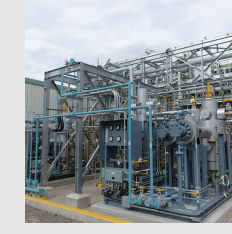
Pilot facility for producing methanol from CO 2
