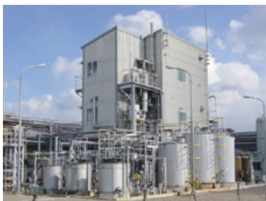
Fig. 15 The HCl oxidation demonstration plant (Plant capacity : 1000t/y)
