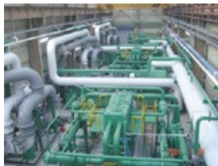
Fig. 4 Inside of Machine Room of O 2 PVSA Plant
