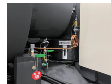
HFO (R1233zd) refrigeration equipment
