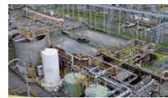
Activated sludge treatment facility
