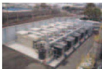
Gas engines installed inside a power and service facility
