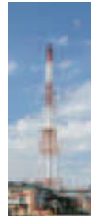
A flare stack for incinerating waste gases
