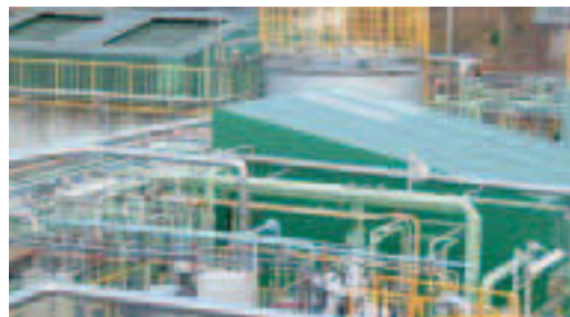
Wastewater storage tanks
