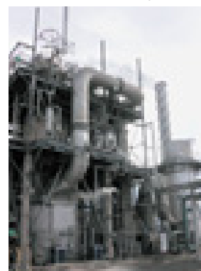
Wastewater incineration facility (Ehime Works)
