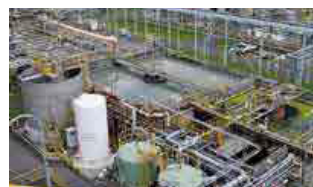
Activated Sludge Treatment Facility
