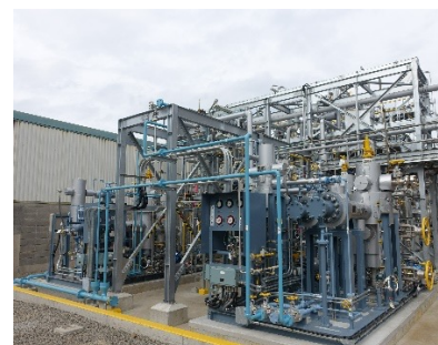
Pilot Facility for Methanol Production from CO 2
