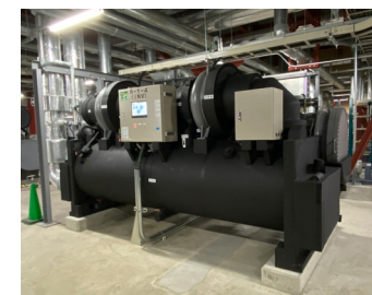
HFO (R1233zd) Refrigeration Equipment
