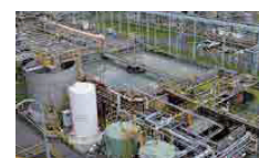
Activated sludge treatment facility
