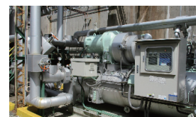
Fluorocarbon refrigeration equipment
