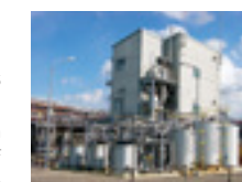
Hydrochloric acid oxidation process equipment
