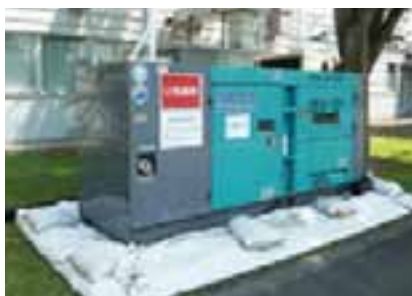
Rental power generator installed at the Tsukuba Research Laboratory
