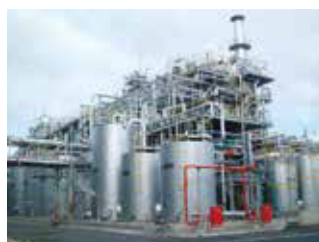
Vapor-phase caprolactam process equipment
