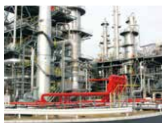
PO-only process equipment
