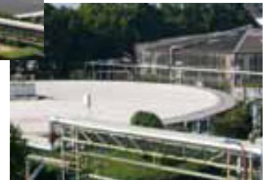
Sedimentation tank covered by white sheeting
