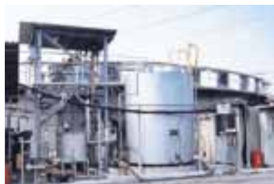
Pilot facility for testing technology for high-density cultivation of nitrifying bacteria
