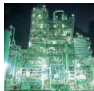
Gas-phase polypropylene manufacturing facility
