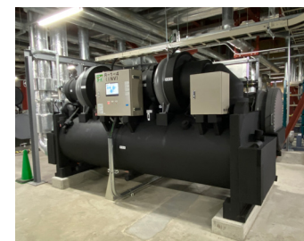
HFO (R1233zd) Refrigeration Equipment
