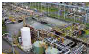
Activated Sludge Treatment Facility
