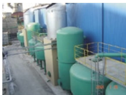
Fig. 5 Outside of Machine Room of O 2 PVSA Plant
