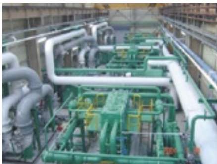
Fig. 4 Inside of Machine Room of O 2 PVSA Plant
