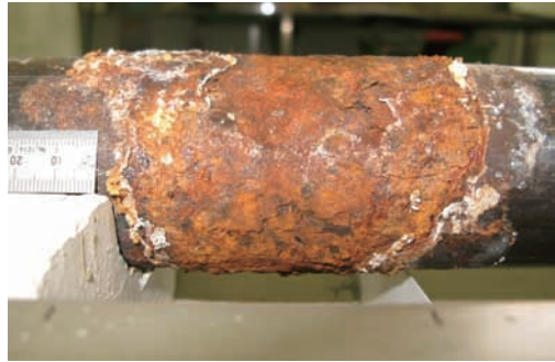
Fig. 13 Corrosion of piping (3rd monitor: 03/2008)
