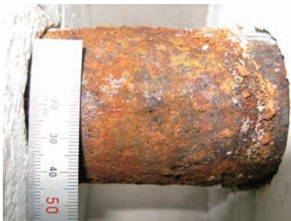
Fig. 11 Corrosion of piping (2nd monitor: 01/2008)
