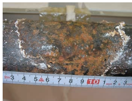
Fig. 8 Corrosion of piping (1st monitor: 11/2007)
